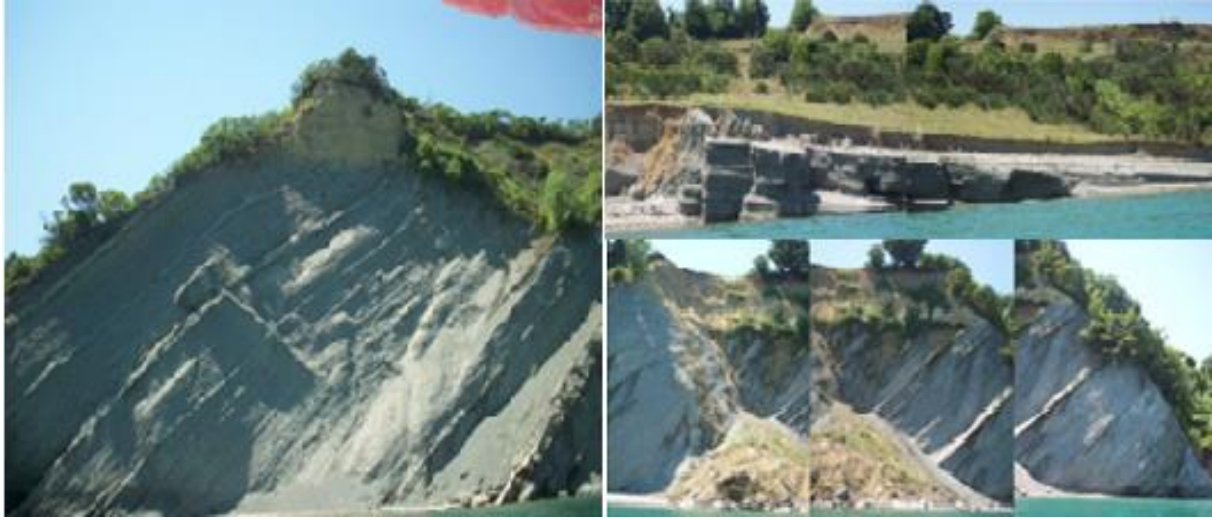
Figure 3. Rock falls occurring at the top of the beddings [cornices] [2]
