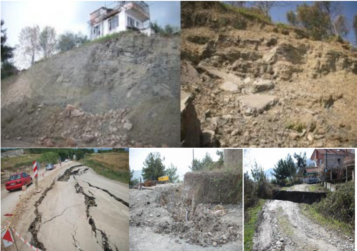
Figure 4. Landslides and damages caused during road construction [2]
