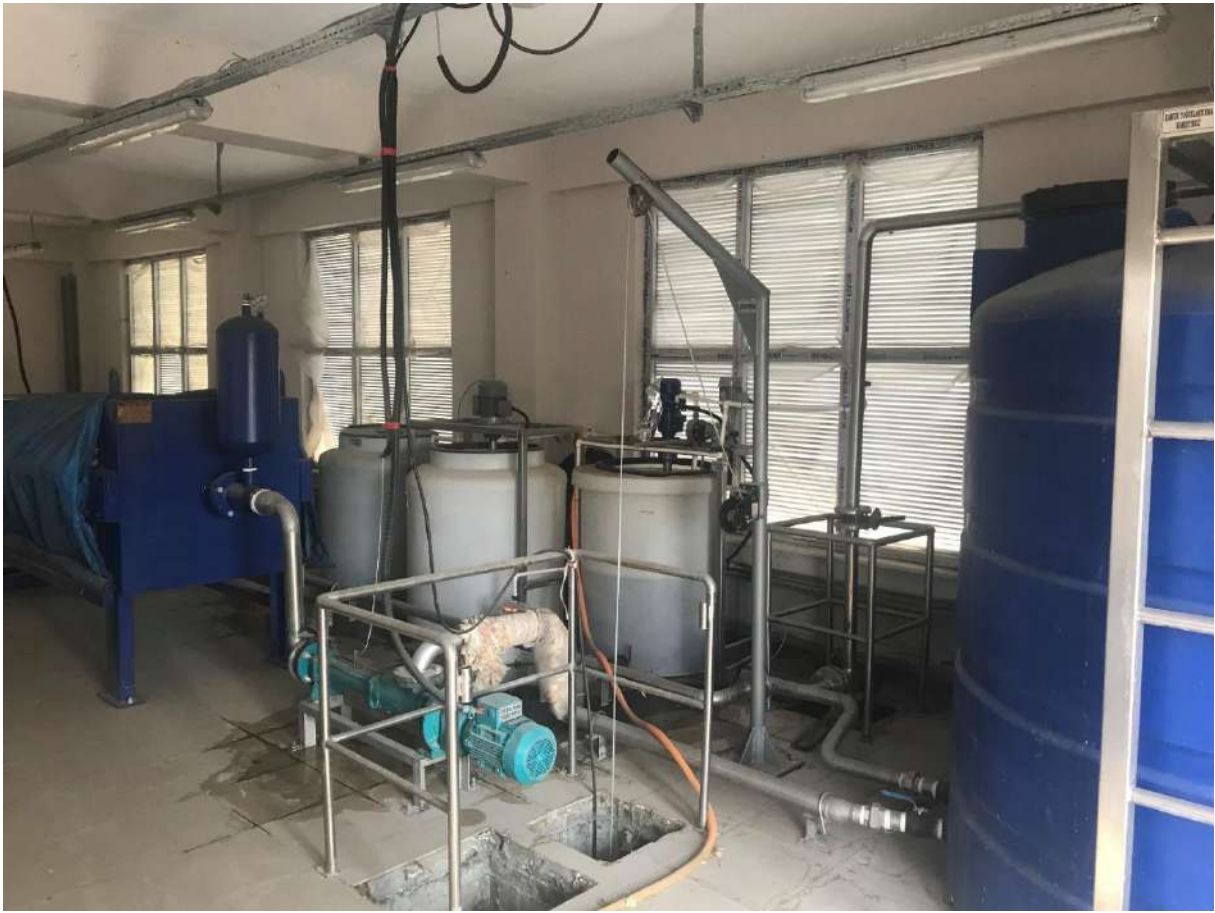
Figure 59. Images from NOHU Sewerage Waste Disposal-3
